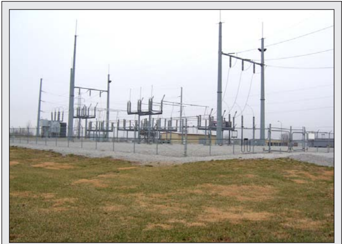
Cleveland recommends perimeter protection so that no one can get into the site undetected. The fence line, entry and egress points are monitored with cameras.
